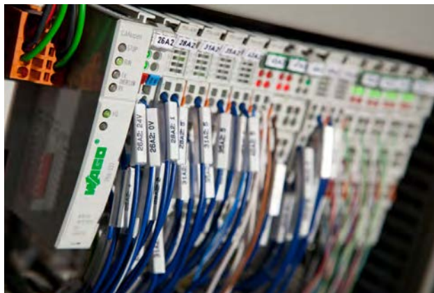
Figure 3: A CANopen Fieldbus Coupler and various I/O modules from the Wago I/O-System ensure communication with the sensors and actuators in the control cabinet (Source: Marc Fippel Fotografie/vor-ort-foto.de)
